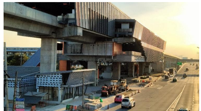
Picture 6: Exterior construction at Min Buri Station on the Orange Line is Currently ongoing
